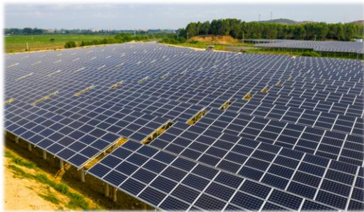
57 acre solar farm
