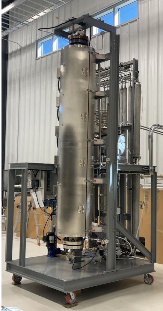
Stand-alone 50kg/day unit on-site
