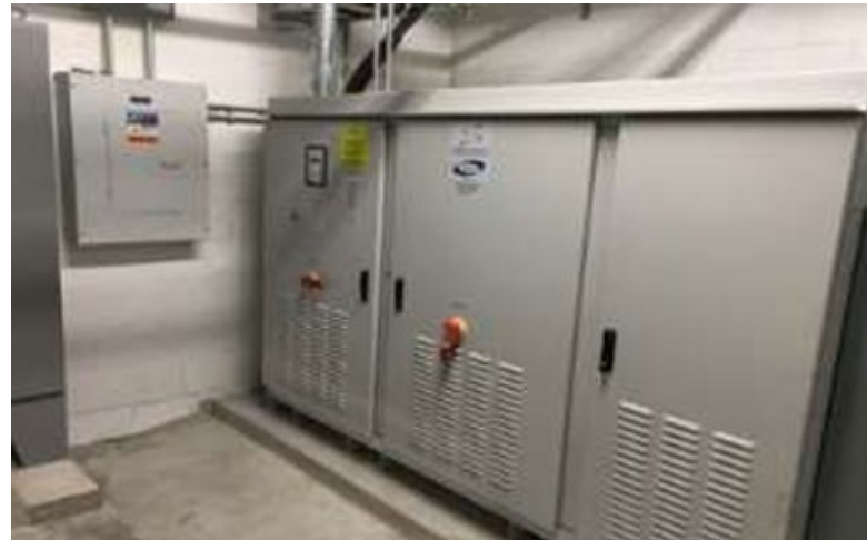
Interior of Inverter Room Showing BIGI250 Photo via CEC Report
