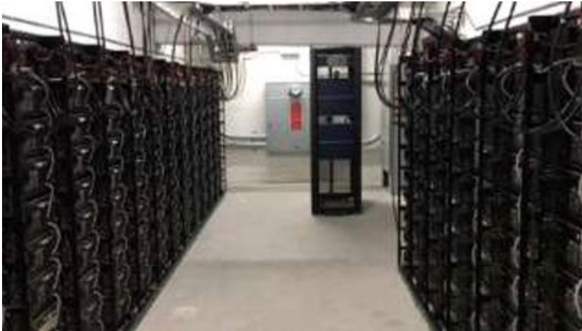
Interior of Battery Room and Electrical Systems Photo via CEC Report
