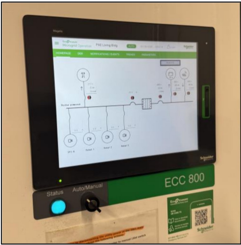
Schneider EcoStruxure Microgrid controller
